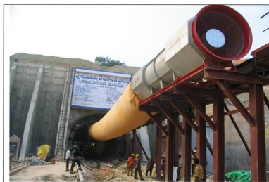
BLOWER PVC DUCTING
